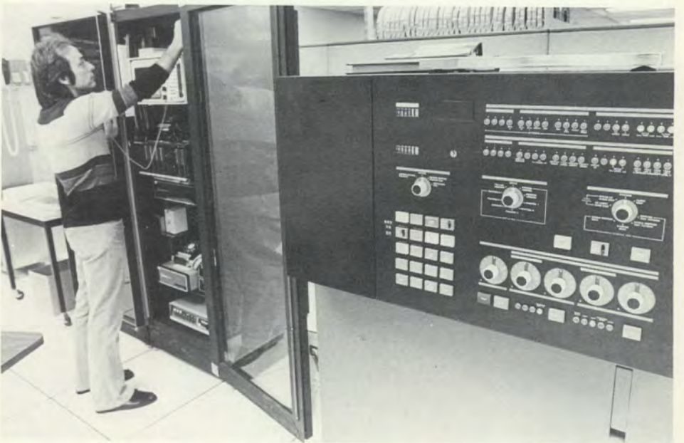
Above, First American's William L. Thiss reprograms channel parameters in one of seven statistical multiplexors handling remote telephone circuits to remote users. Below, Don Rice of Unigard Insurance patches a data scope into one of numerous telephone circuits to monitor the line in First American's service bureau environment; at right is the minicomputer serving as "traffic cop" between the main computer and telephone circuits.
