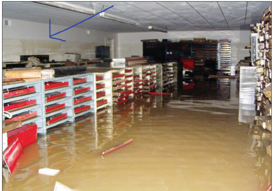
▲ Metropolitan’s Title Plant, showing the water line from the flood.
